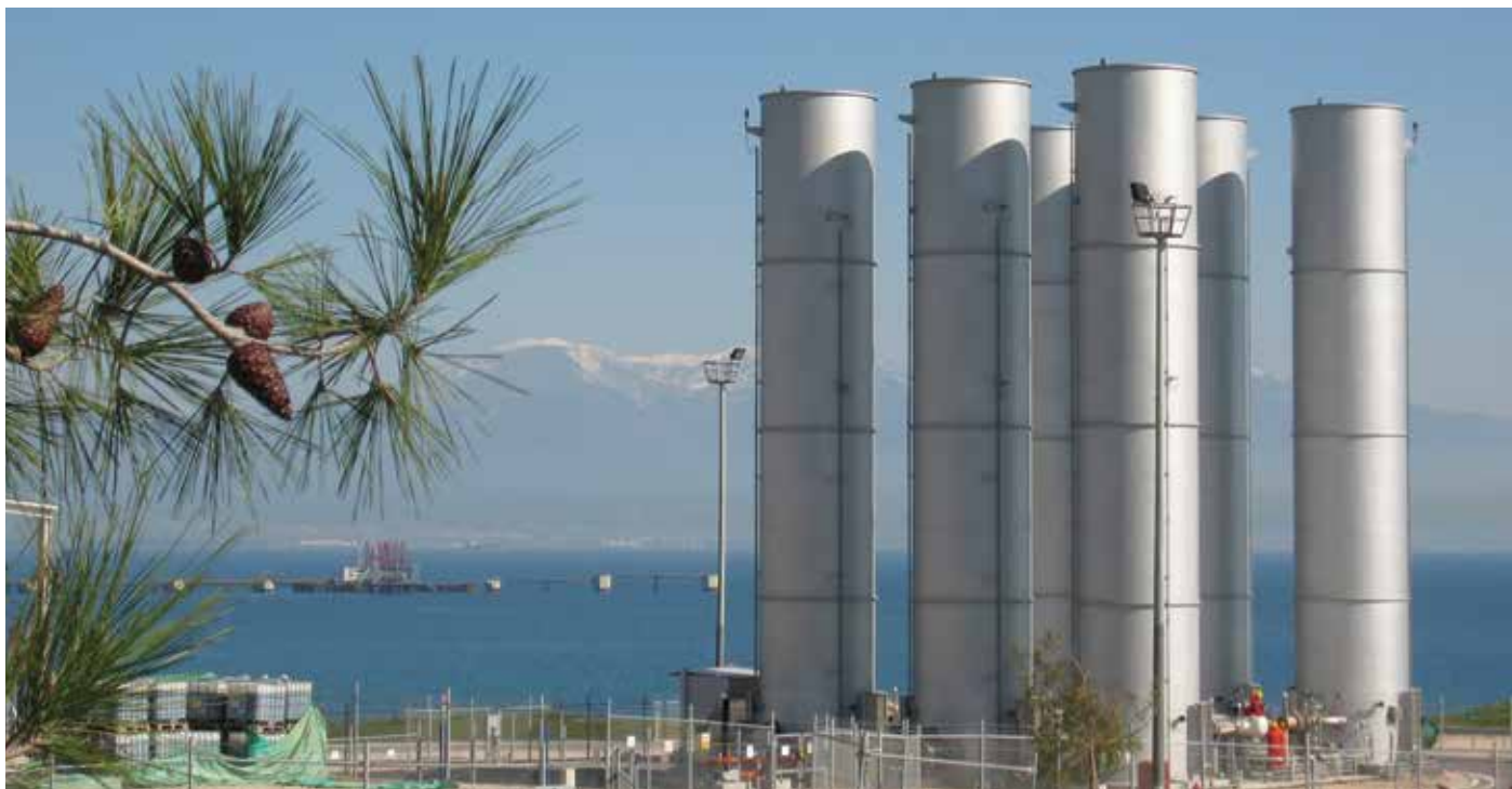
MULTI-STACK MARINE VAPOR COMBUSTION SYSTEM
