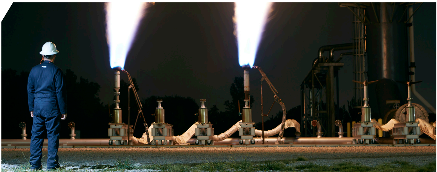
JZ Indair First Stage Burners
