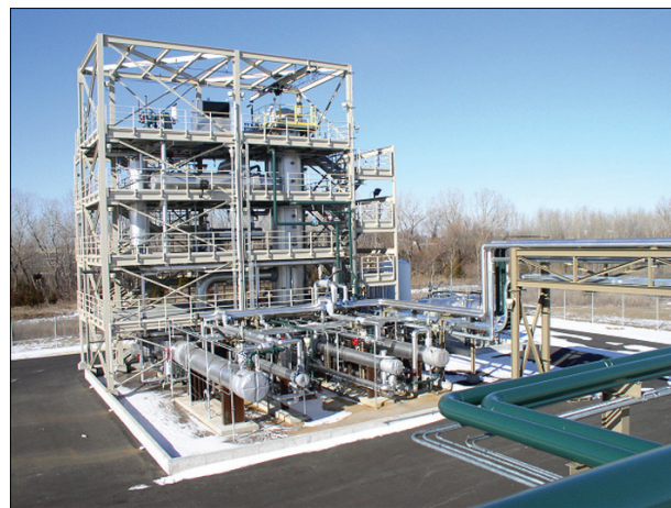
Figure 8 – A complete CO 2 capture pilot unit is available for testing a wide variety of solvents
