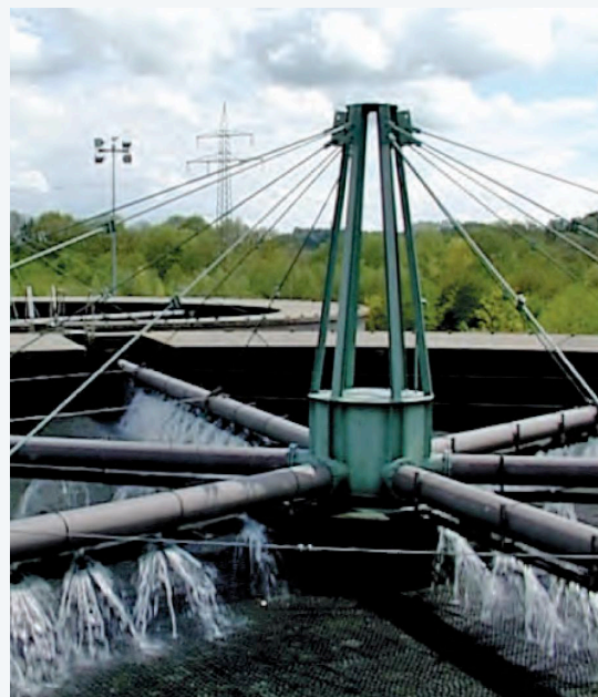
WATER TREATMENT FACILITY
