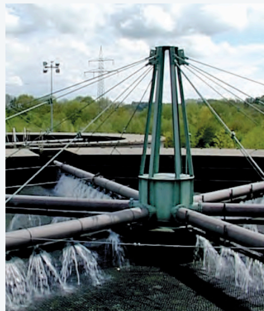
WATER TREATMENT FACILITY
