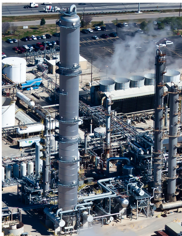
Figure 1. This 28 ft (8.5 m) dia. x 330 ft (100 m) tall propane/propylene splitter was retrofitted with SUPERFRAC® XT trays.
