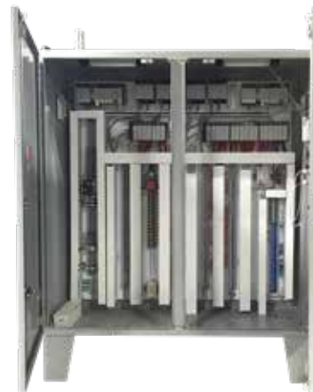
BMS and Control Panels
