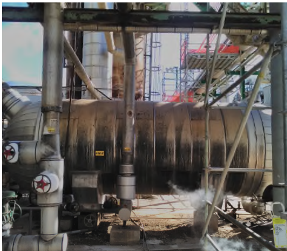
Figure 4. Elevation view of product separator #106F at Enid plant, showing vapour outlet.
